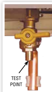
FIGURE 23. GAS PRESSURE TEST POINT
